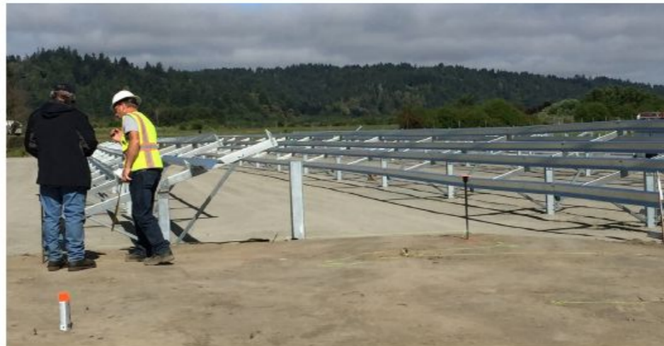
Workers installing the racking for the Blue Lake Rancheria's 500-kilowatt solar system in June 2016. The solar system is a cornerstone of the tribe's low-carbon community microgrid project.
