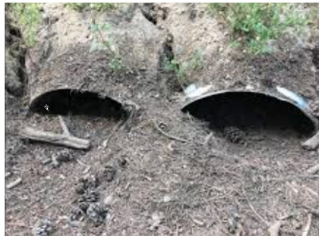
Figure 12. Clogged Culverts Raise Flood Concern in Black Forest (KRDO News)
