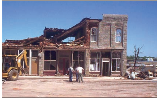
Surveying the damage in Stockton, Mo.
